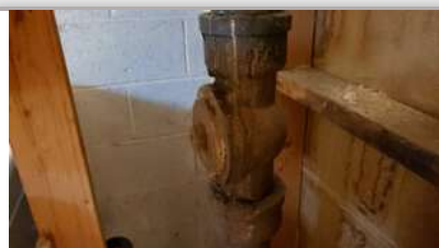
MAIN WASTE LINE CLEANOUT
