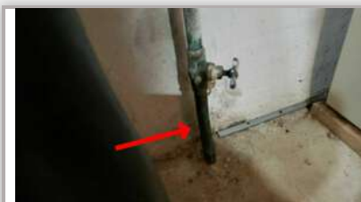
MAIN WATER LINE
