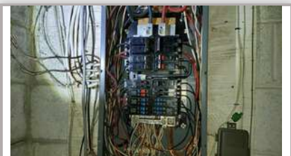
ELECTRICAL PANEL INTERIOR
