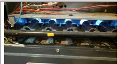
FURNACE BURNERS IN OPERATION
