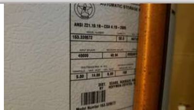
WATER HEATER DATA PLATE
