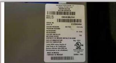
EVAPORATOR DATA PLATE
